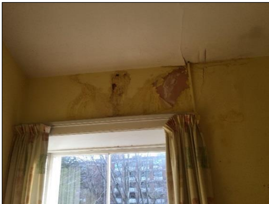
Figure 9. Example of water ingress (Source: Molloy & Associates Conservation Architects)
