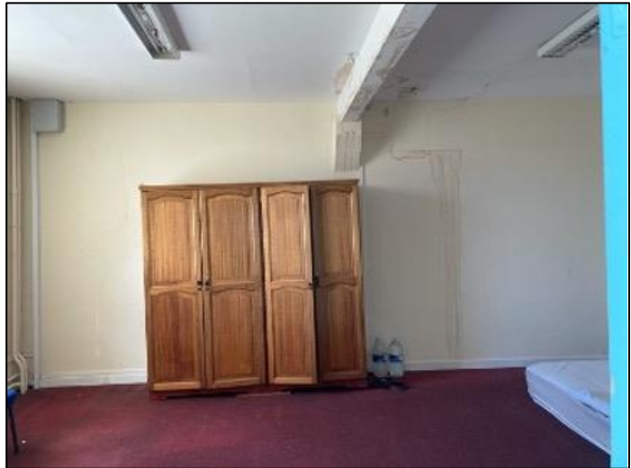
Figure 8. Amalgamated room, with evidence of water ingress and exposed services
