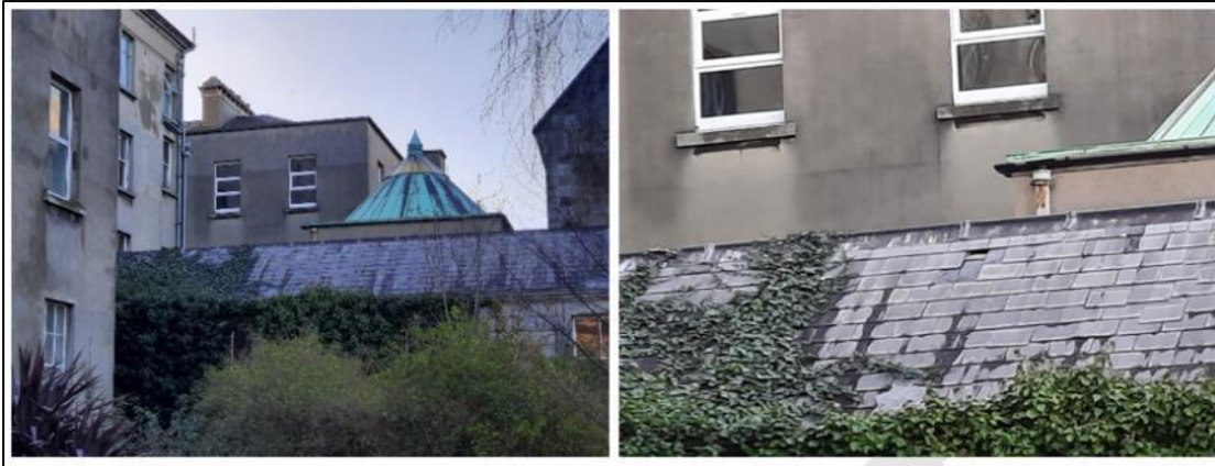
Figure 8.35: PRF (broken Tile) on the east face of the Chapel (Source: DNV).
