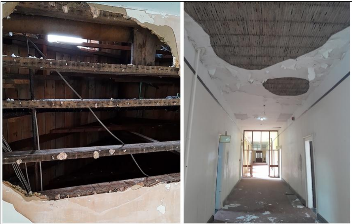
Figure 8.31: Images showing the level of disrepair of the ceilings and attic floor in Tabor House. Daylight can be seen through a skylight in the roof in the left-hand image (Source: DNV).
