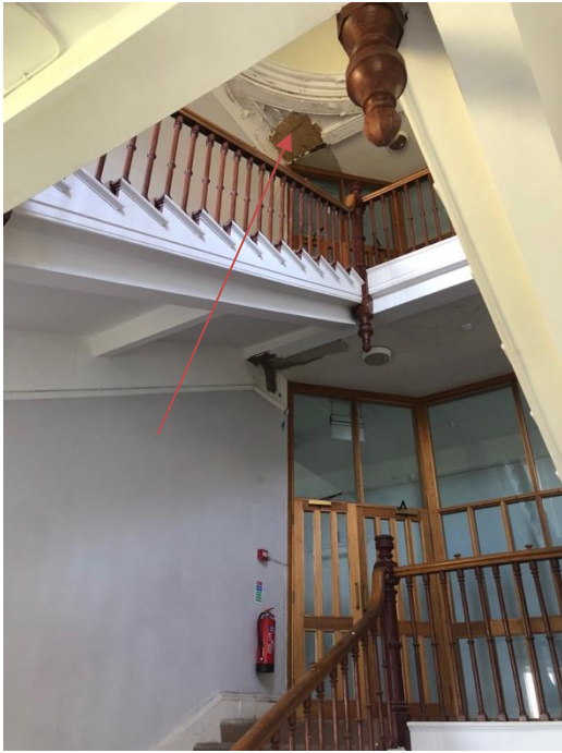
Plate 191: Damage to ceiling above main stairwell.
