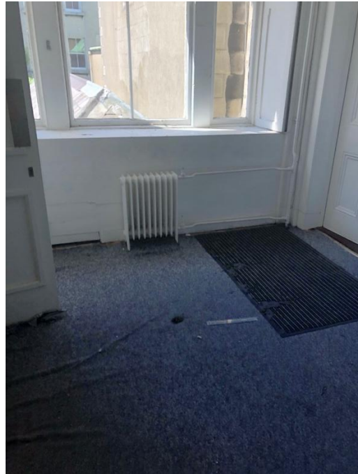
Plate 267: Damage to ceiling and wall fabric due to water ingress.
