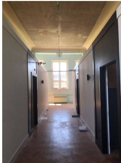
Plate 318: View within upper floor facing north. Mould growth evident on coppered ceiling. Note: Low partition walls are part of a recent, temporary installation.
