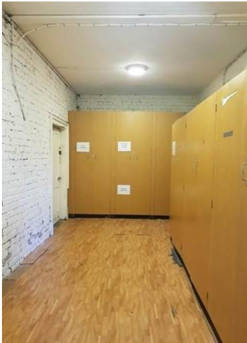
Plate 228: Plant room at basement level. Exposed brick, painted finish.
