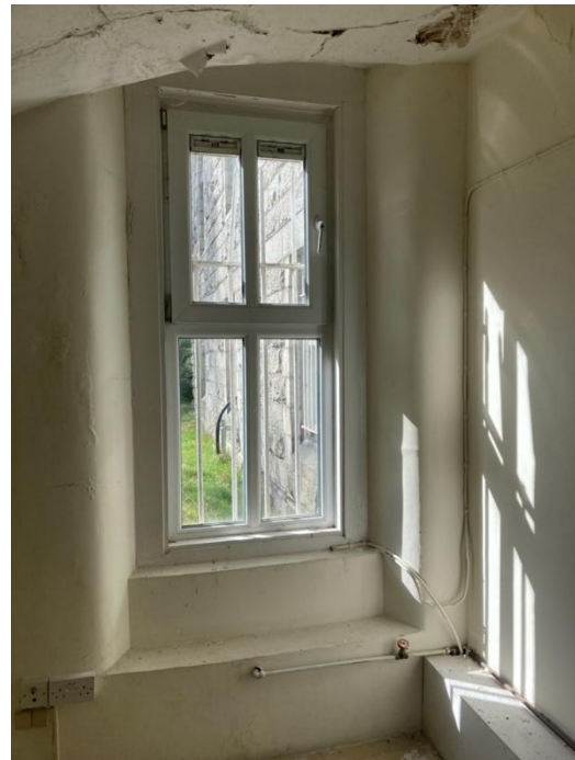
Plate 233: Contemporary uPVC window on lower ground floor. Beneath main entrance. Note deterioration of ceiling fabric indicative of water ingress through exterior steps.
