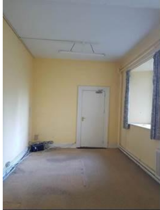
Plate 299: Evidence of water ingress at base of wall.
