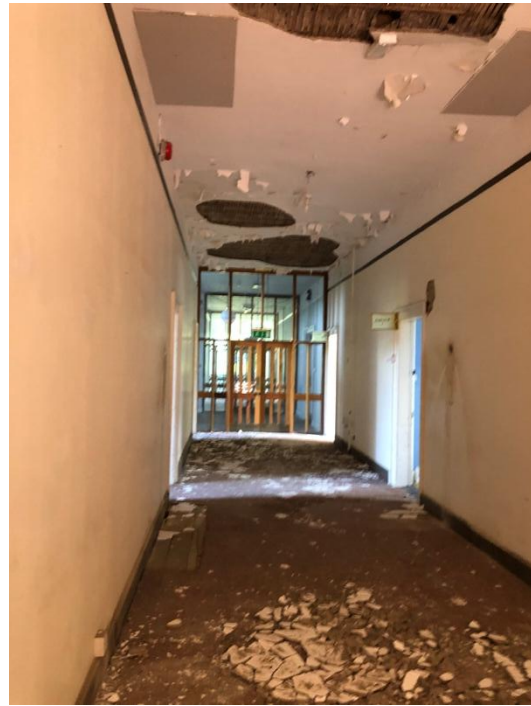
Plate 203: Entrance level corridor with later cross-corridor fire screens. Collapsed ceiling fabric due to water ingress in view.
