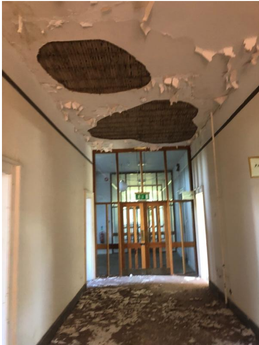
Plate 202: Entrance level corridor with later cross-corridor fire screens. Water ingress damage to ceiling fabric.
