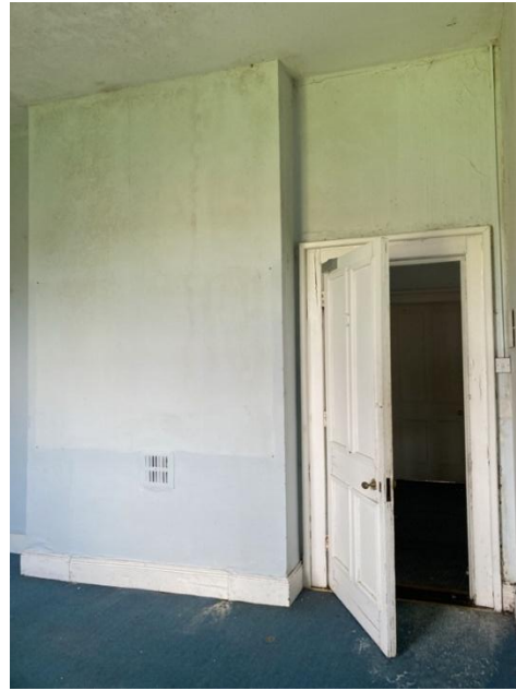
Plate 263: No chimneypiece. Original joinery. Staining of ceiling suggestive of water ingress.
