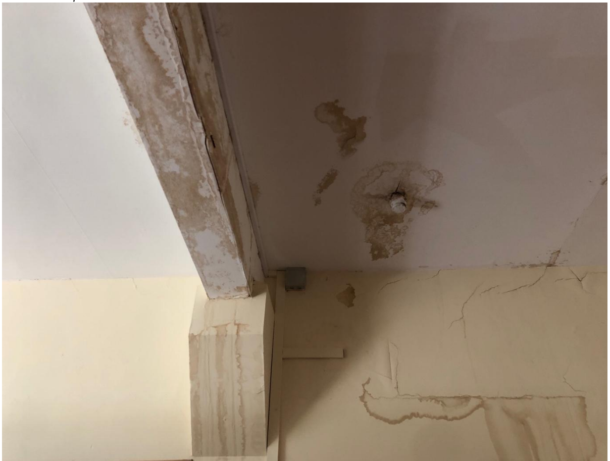
Plate 113: Amalgamated room, with beam supporting structure on level over. Evidence of water ingress. Exposed services. No chimneypiece or historic plasterwork.
