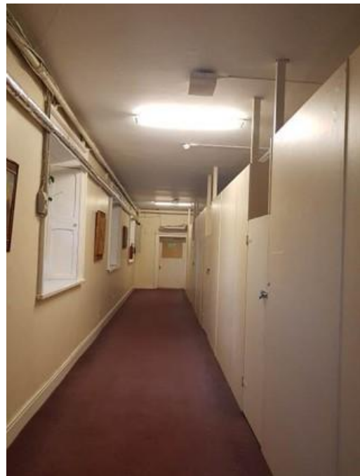
Plate 229: Basement corridor with original window joinery.
