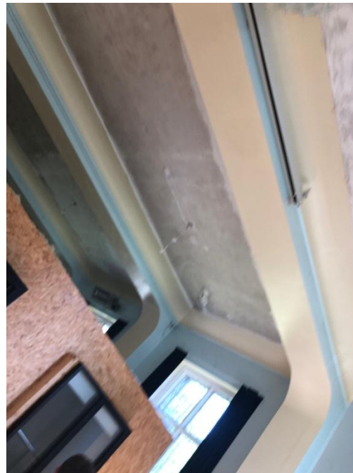
Plate 324: Ceiling showing some signs of water damage
