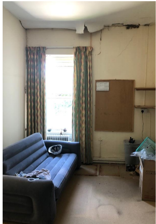
Plate 123: Sample room within vertical extension above main house. Note water ingress from breaches at roof level
