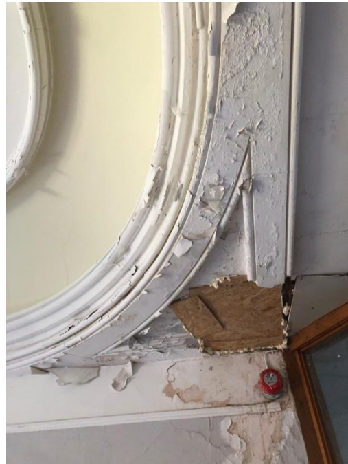
Plate 192: Flaking paint and staining of ceiling due to water ingress.
