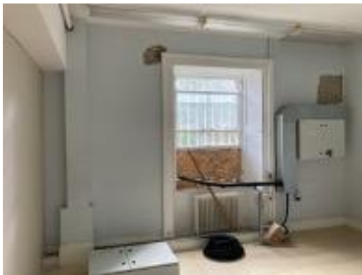
Plate 224: Ad-hoc nature of services threaded through original fabric and temporary weathering.
