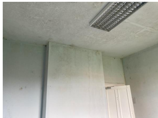
Plate 273: Mould growth evident on wall and ceiling surfaces.
