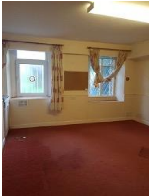
Plate 133: Dormitory at lower ground floor level. Note water ingress
