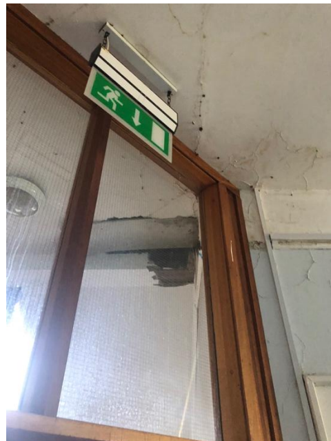
Plate 265: Water ingress damage from roof impacting second floor corridor ceiling
