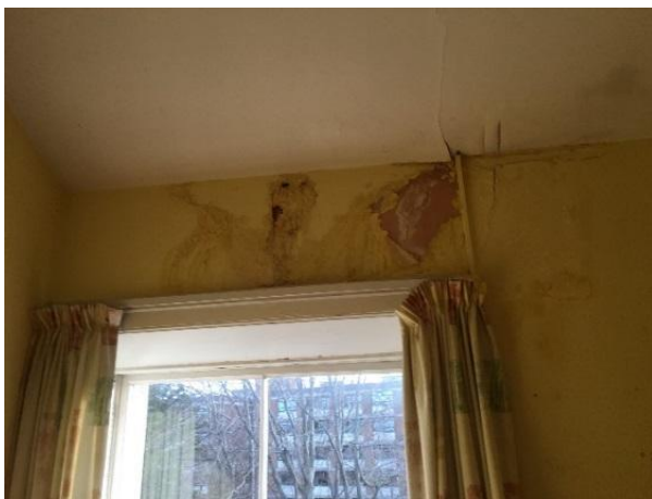
Fig. 35 Example of decay due to water ingress from breaches in roof coverings, at 2 nd floor (later intervention) level
