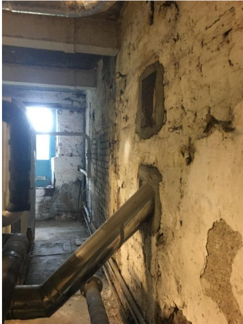
Fig. 33 Former kitchen to northwest at basement level, with original masonry and floor flags evident. Note concrete downstands for concrete floor plate supporting entrance level above.
